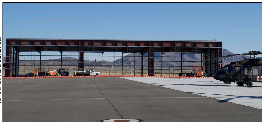
This photo shows ongoing construction of the Nevada Army Aviation Support Facility's UH-60 hangar on the north end of the Harry Reid Training Center in Stead, Nev., Sept. 20, 2024. The 6,355 square foot storage hangar will provide room for three UH-60 Black Hawks.
